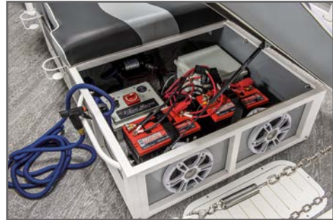
Battery Control Center and Washdown Station
